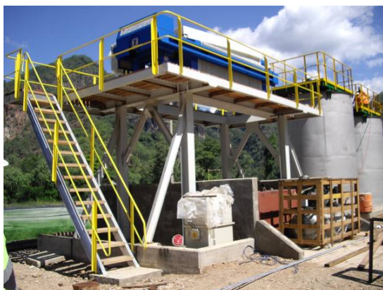
Fig 2: Filter Press and neutralisation Plant
