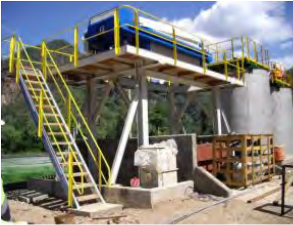
Figure 5. Filter press and neutralisation plant
