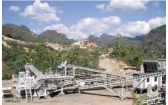
Figure 6. Refurbished crusher at Wetar
