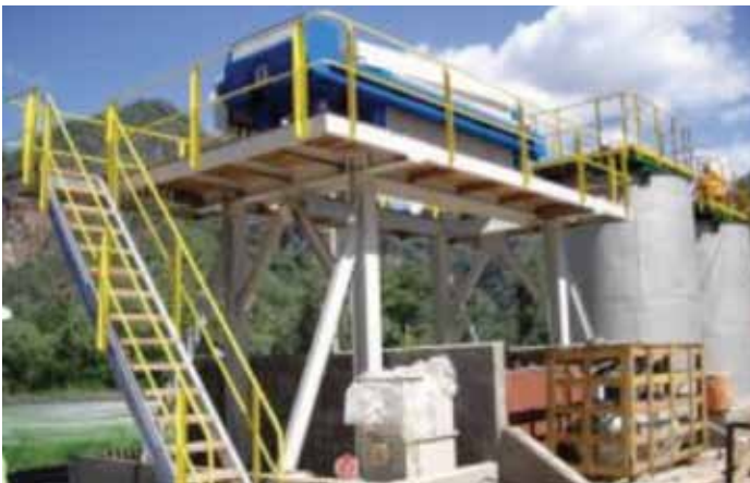
Figure 5. Filter press and neutralisation plant
