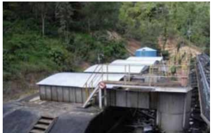
Figure 8. Covers on the SX plant
