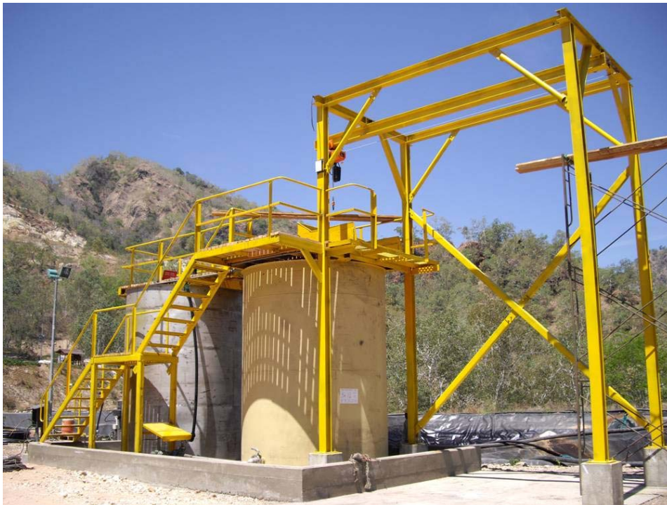
Figure 3: Acid neutralisation plant
